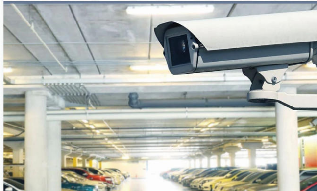
Provision for CCTV in Parking Area
